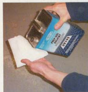
1. Start out by thoroughly cleaning the areas where the mat will be applied. We used DuPont Prep-Sol, but any good cleaner/degreaser will work fine.
